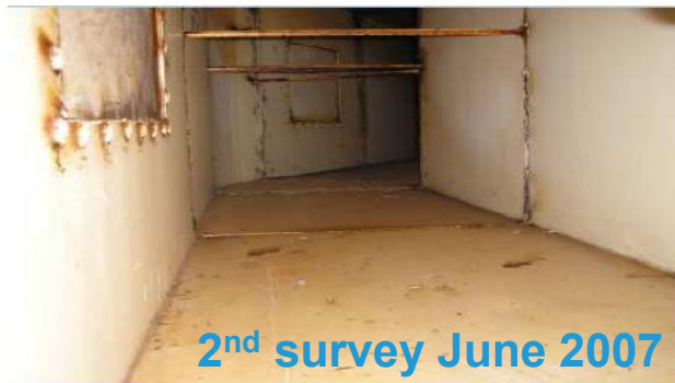
Crew Galley, UVC retrofitted end of 2004
