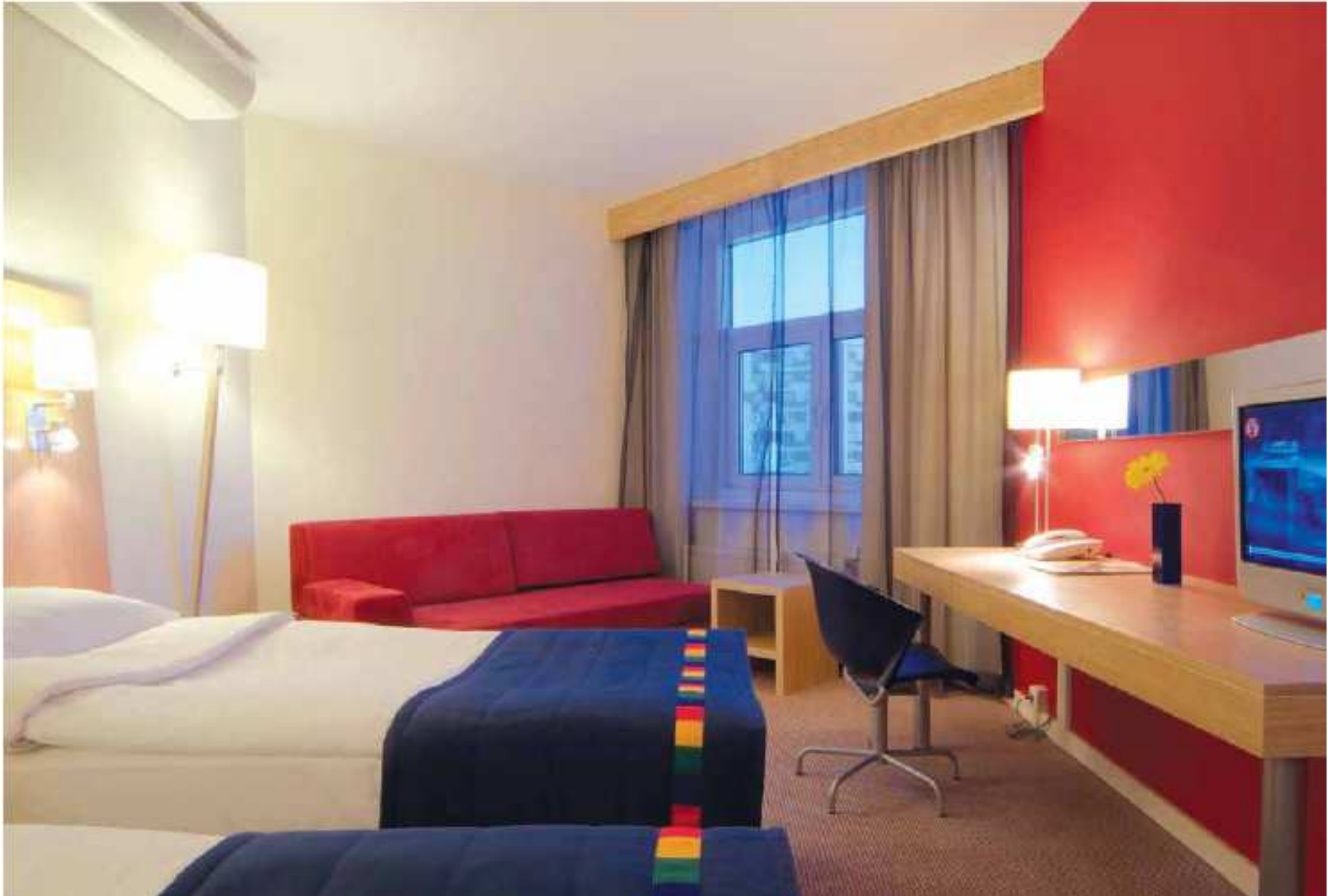
Halton Chilled Beams Applications for Hotels
