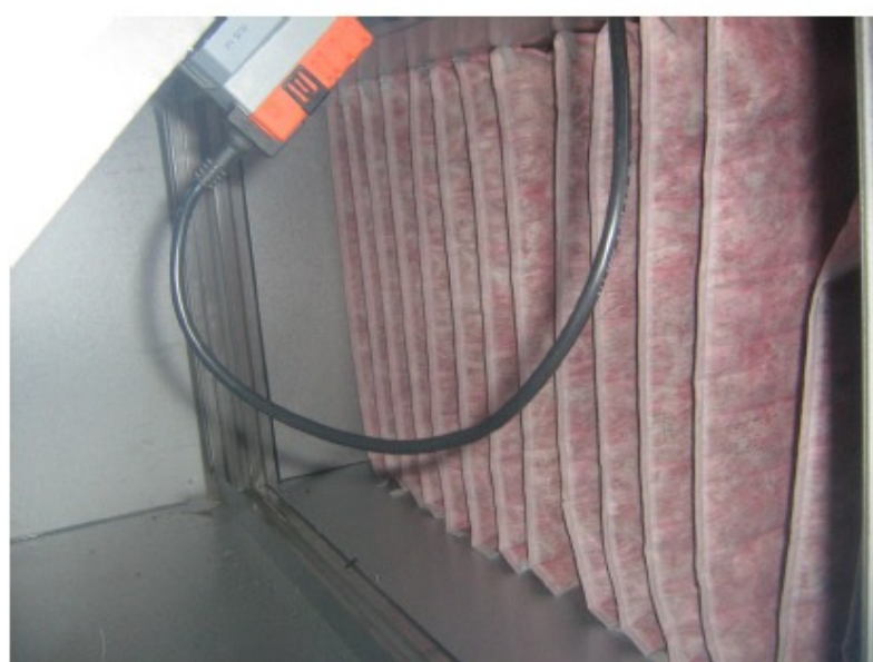
The heat exchanger filter package 30.11.2010
