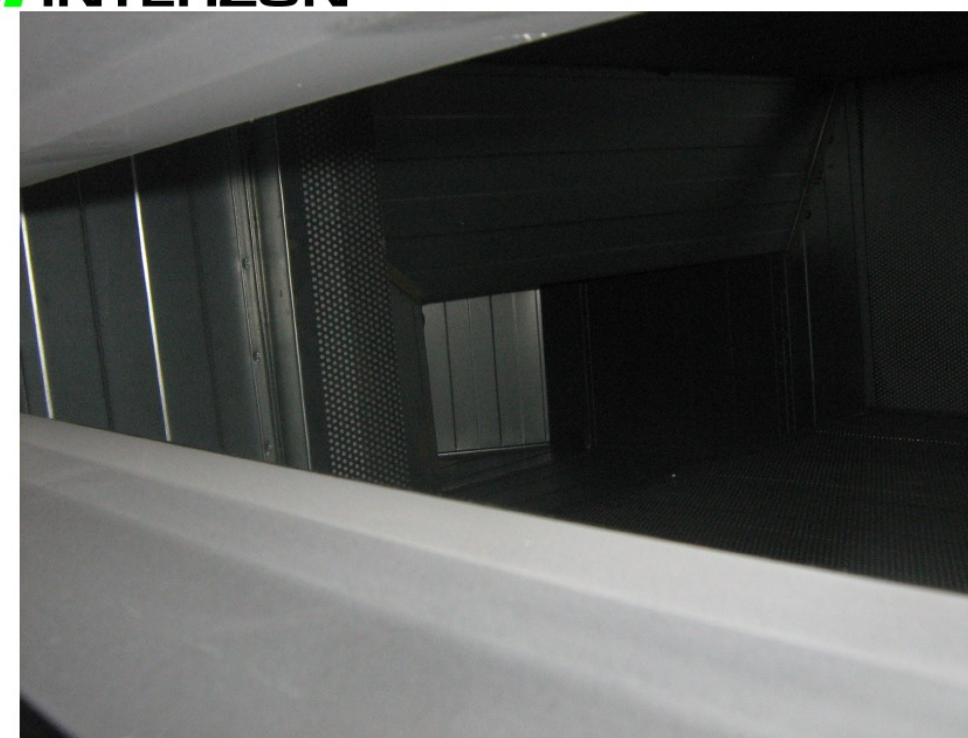
The grease duct just before the heat exchanger.
